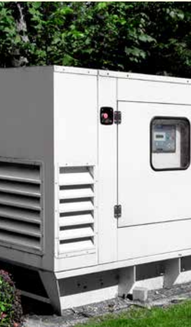
Generator or battery backup
